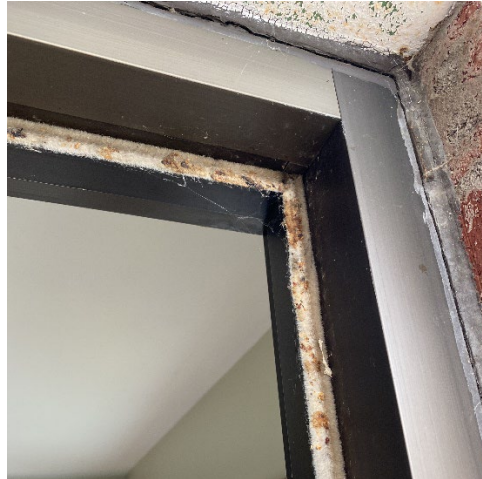
Weather stripping was present around the head and jambs of the doors, however they were quite compressed and dirty.
