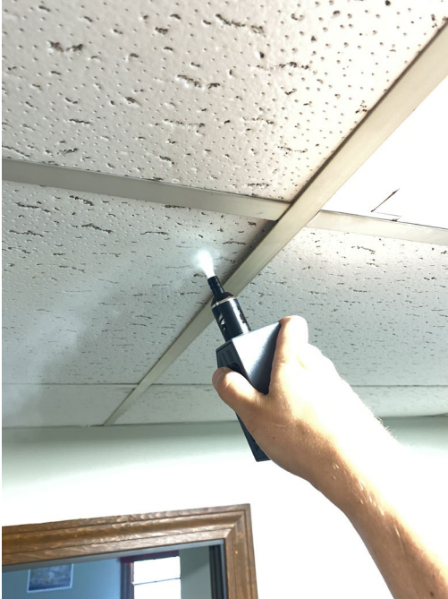
Difficult to see in the photo, but fog is being blown down and to the left from the air movement coming through the corner of the ACT where it is not fitting tightly to the grid.
