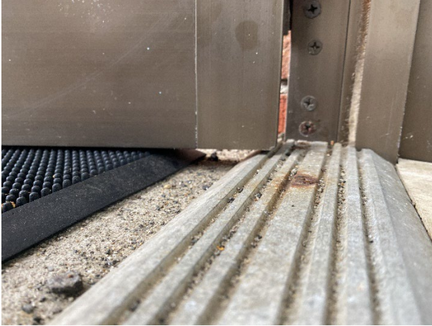
A view of the bottom of these doors, not brush sweep or weatherstripping is present at the threshold.
