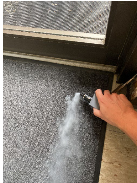
Fog shows that a strong current of air is present at the bottom of the door. This was consistent at both exterior vestibule doors.
