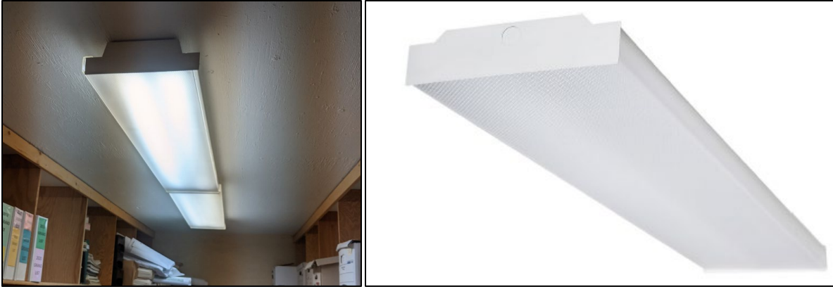
Figure 10: T12 wraparound fixtures in downstairs vault (left) and potential LED replacement (right)
