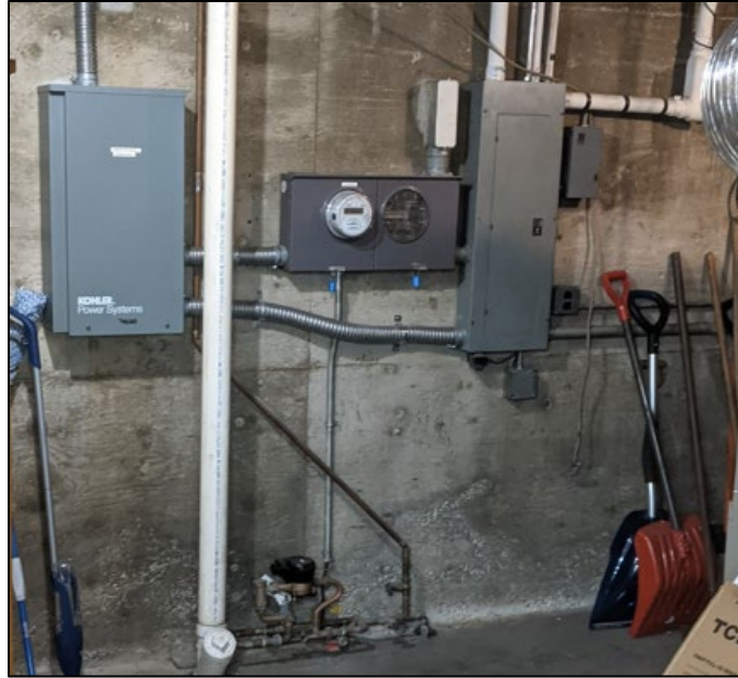
Figure 13: Electrical meter and panel
