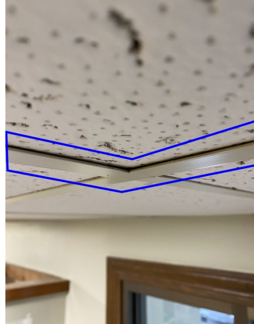
An example of the small gaps present around the ACTs, they do not create an air-tight seal to the grid.
