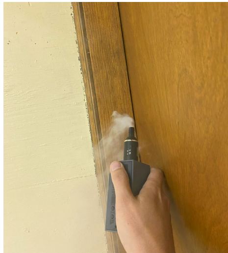
Air was consistently observed flowing around this door, as no weather stripping was present.
